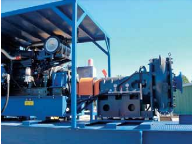
The booster station used in the new Carolina Sand system.
